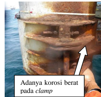
Gambar 18 Tampak dekat clamp Line B [8]
