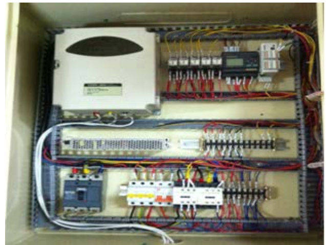
Gambar 6. Panel control pengujian
