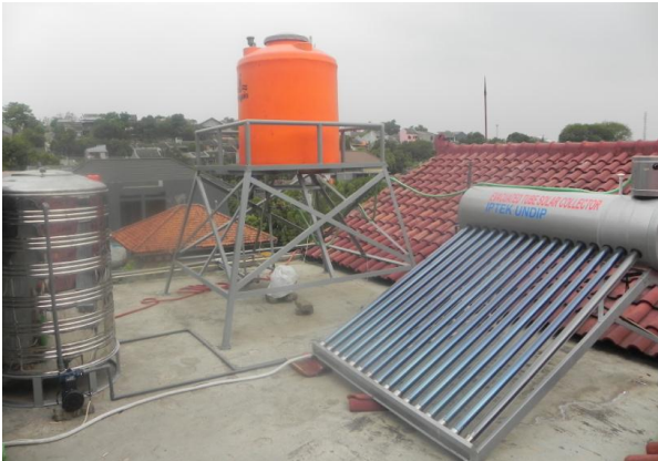
Gambar 13. Instalasi model sistem evacuated tube solar water heater
