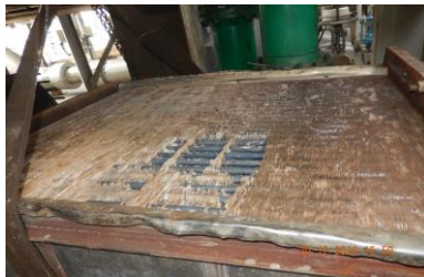
Gambar 10. Kerusakan Pin Tube Intercooler
