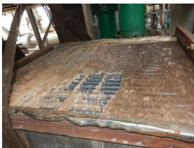
Gambar 10. Kerusakan Pin Tube Intercooler
