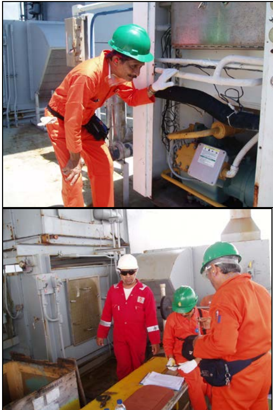
Gambar 2: Kompresor , AHU, Mixing HVAC Kakap Field Star Energy Natuna
