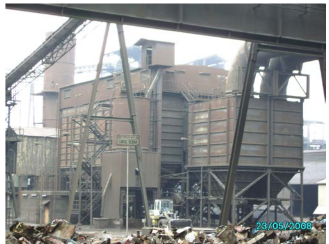
Gambar 4. Mixing Chamber dan Filter House (Sumber: PT. Krakatau Steel, 2008)
