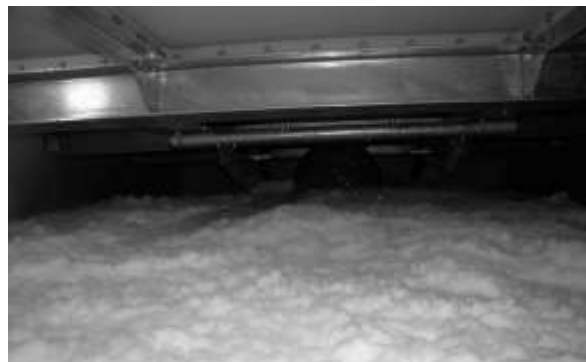
Figure 9. Appearance inside ice storage tank at fully accumulated state ( IPF = 45\% )
